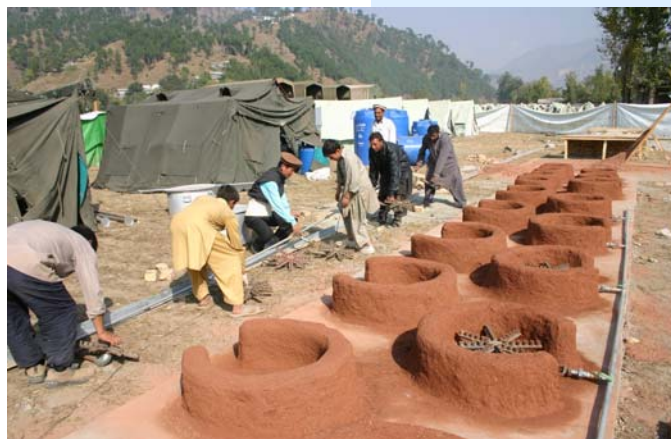
The South Korean Emergency Relief Centre building stoves for a kitchen. Bassian camp near Balakot in NWFP. / UNHCR / B. Baloch / October 2005
